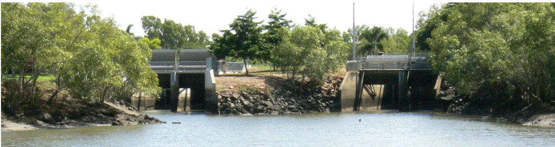
Figure 2.13 Woolcock Street Drainage in a Tidal Setting
