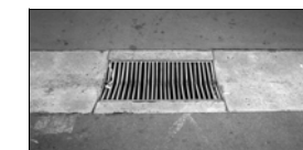
Grates used to prevent entry of gross pollutants
